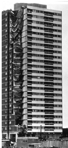
Figure: Damage caused by explosion
